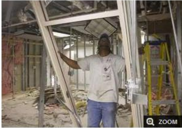
Joseph Glann of RD Johnson Construction Inc., removes an old doorway while completing the demolition of old offices on Wednesday at Lee Memorial Hospital. / AMANDA INSCORE/THE NEWS-PRESS
